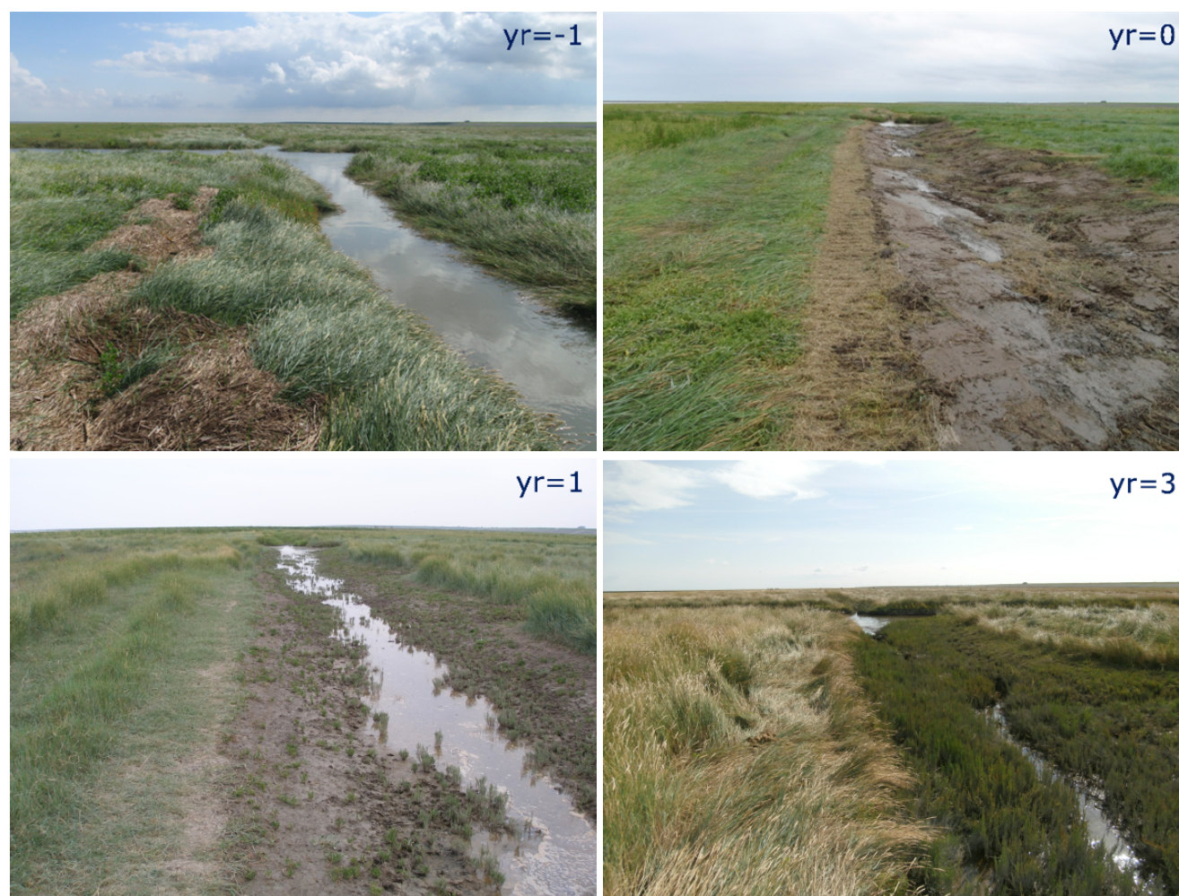
Figure 9. The effect of the partial filling of a collector drain in the salt marsh of Negenboerenpolder, the Netherlands, illustrated by a time series from the year before the filling (yr = -1) until three years thereafter (Photos: W. van Duin).
